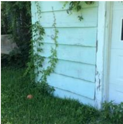
- Grounds - Rotten wood on Shed
