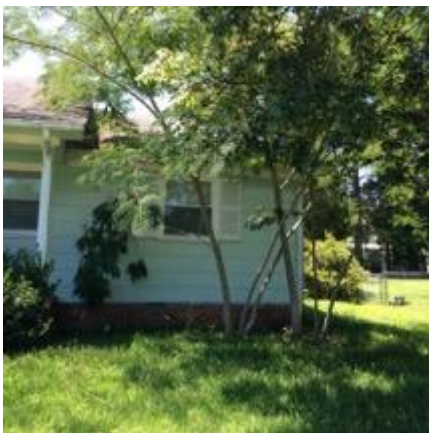
- Grounds - Tree touching roof
