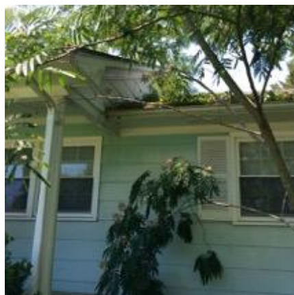
- Exterior Walls - Recommend cleaning gutters and replaced rotten fascia board
