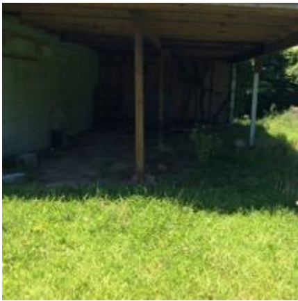
- Grounds - Recommend cleaning shed
