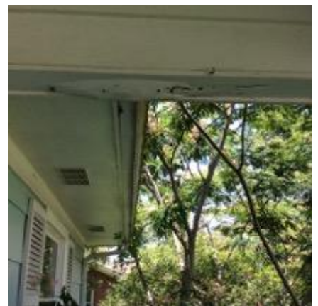
- Exterior Walls - Recommend replacing rotten wood
