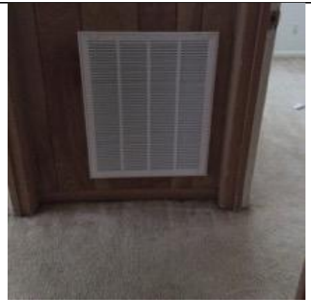
- HVAC Filter and Grates Cleaned? -
