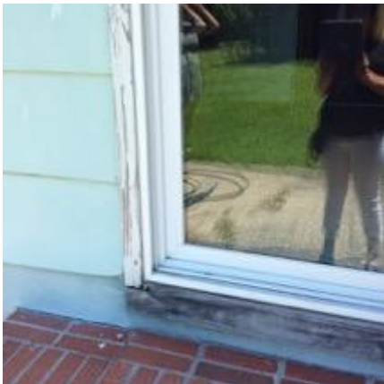
- Exterior Walls - Rotten wood
