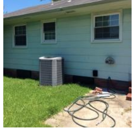
- Exterior Walls - Recommend removing items from property
