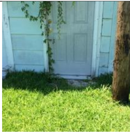
- Grounds - Recommend replacing rotten wood on exterior of shed
