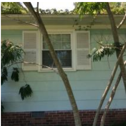
- Exterior Walls - Shutters need to be painted
