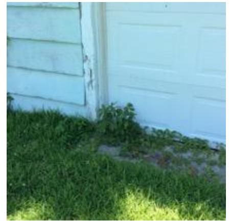
- Grounds - Rotten Wood on Shed
