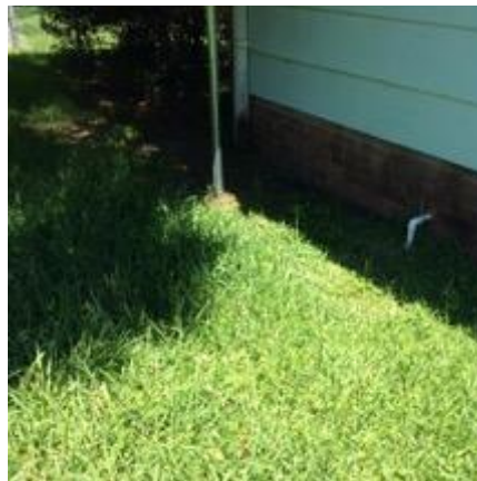
- Exterior Walls - Recommend replacing down spout
