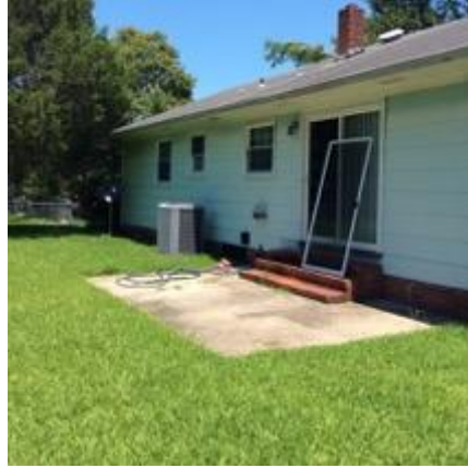
- Exterior Walls - Recommend repairing screen door
