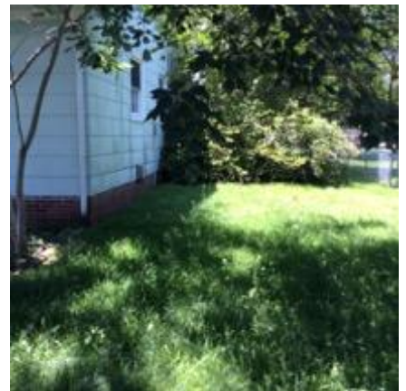
- Exterior Walls - Recommend replacing down spout
