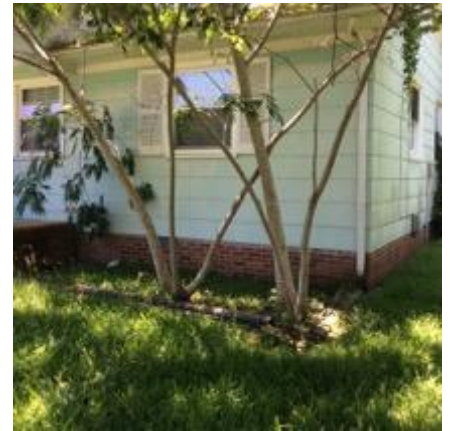
- Grounds - Recommend Tree Away from home or remove tree completely.
